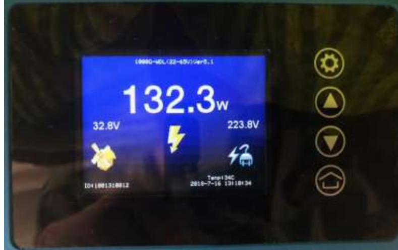
Main „Power View“ display during normal operation
